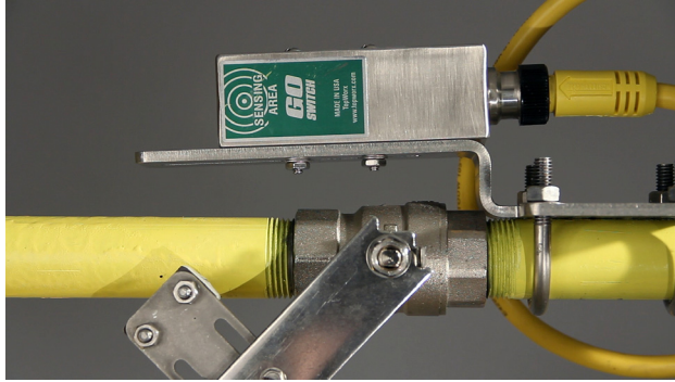
Figure 7-16. Safety Shower Valve in the Activated Position.
