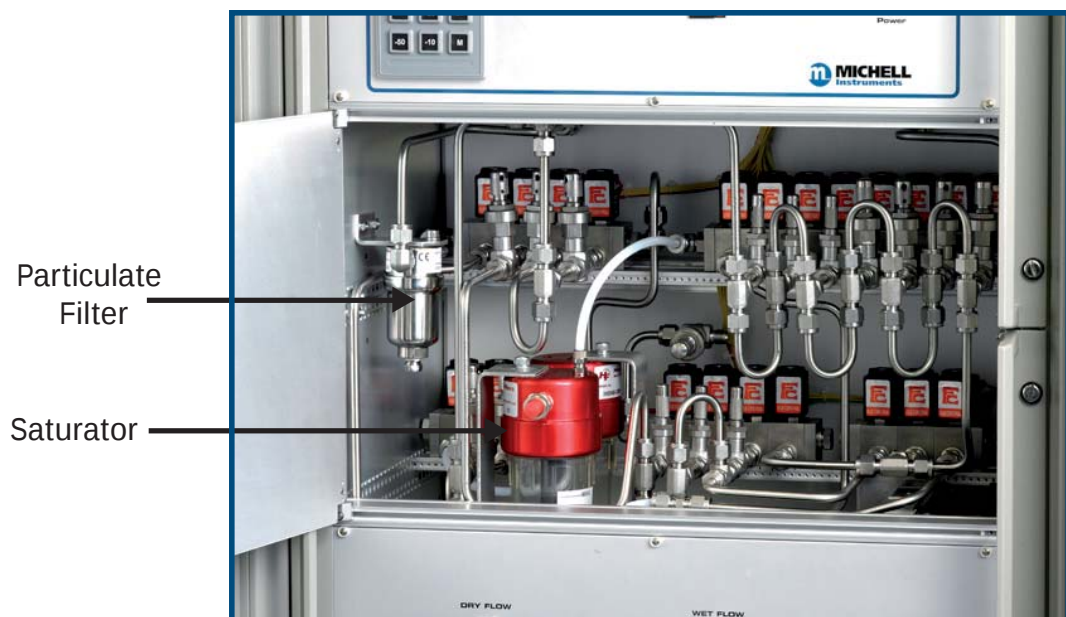
Figure 3 Saturator and Filter Location
