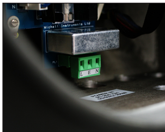
Figure 2 Power Connection Connector
