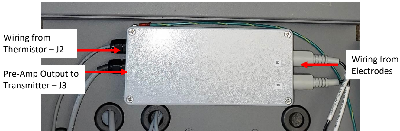
Figure 10. Pre-amplifier located behind the wet panel.
